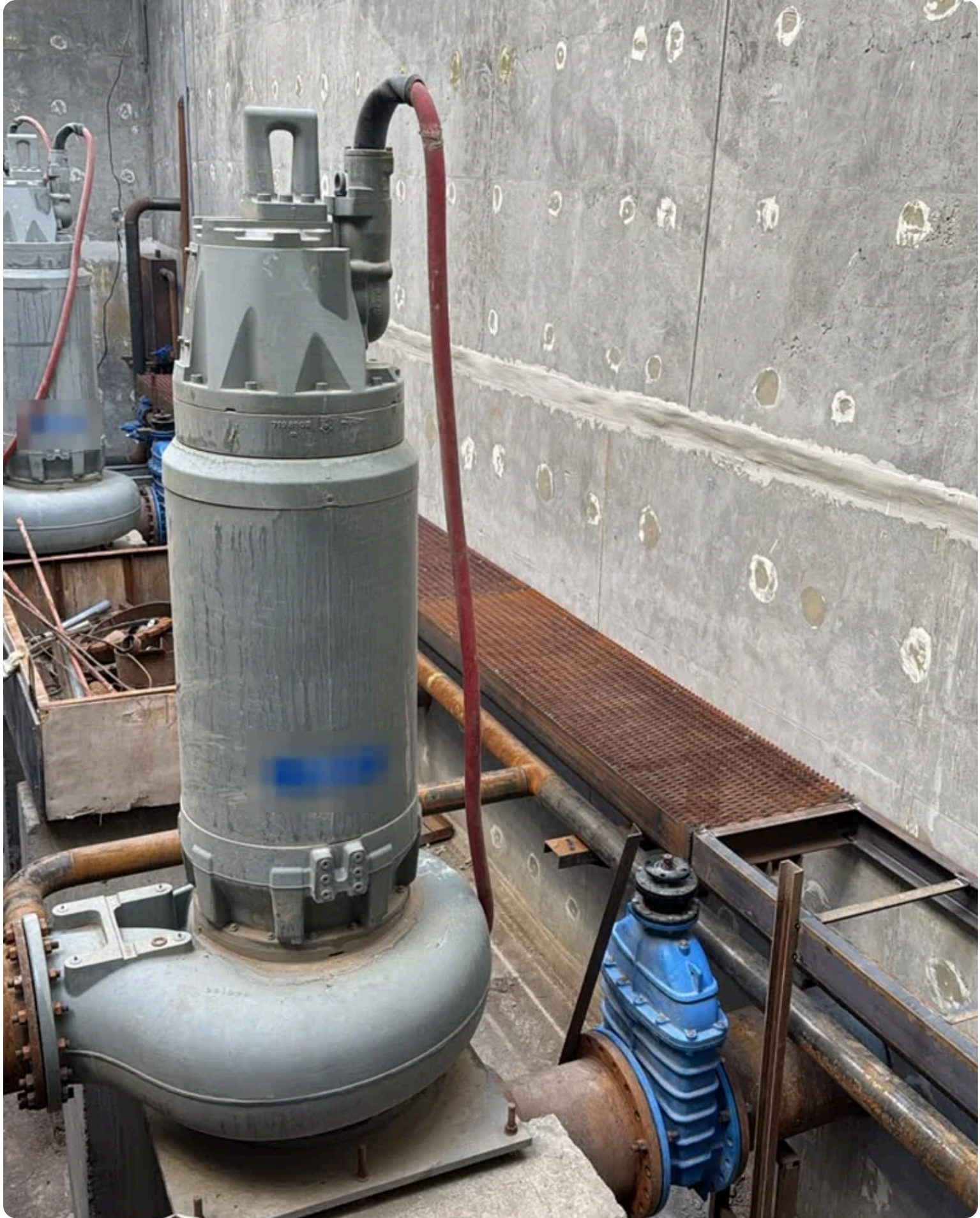
One of the submersible pumps at Pavlodar River Port. The red cable is its existing supply cable; brand labels are blurred. Photo: taken on site.
